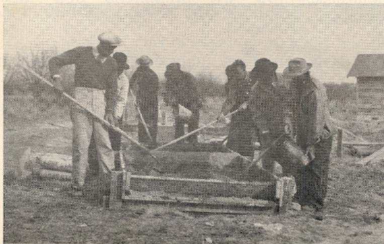
A Group of Farmers Mixing Concrete to Pour Foundation for the Low Cash Cost House at the Eleventh Farm and Home Week, Tuskegee Institute, Alabama.
